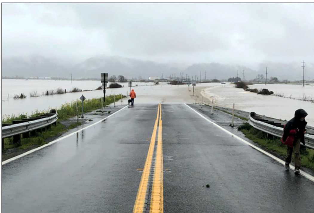
Figure 16. In February 2019, heavy rains brought flooding to the Eel River Valley, closing Highway 211, isolating the town of Ferndale and causing the death of one person. Source: California Department of Transportation.
